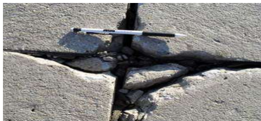
Figure 48 Medium Severity Corner Spalling
