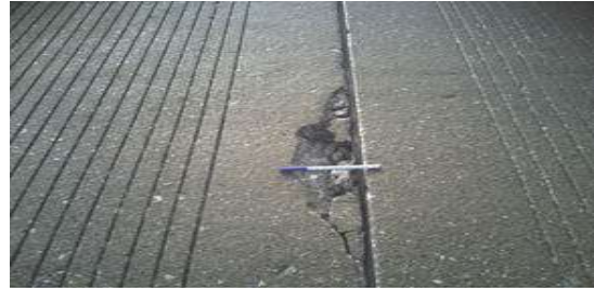
Figure 45 High Severity Joint Spalling
