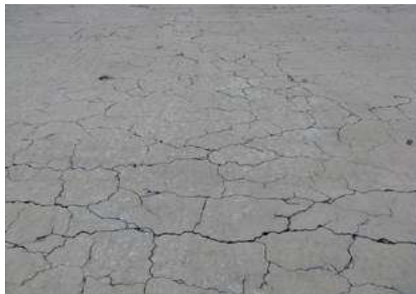
Figure 38 Medium Severity Scaling
