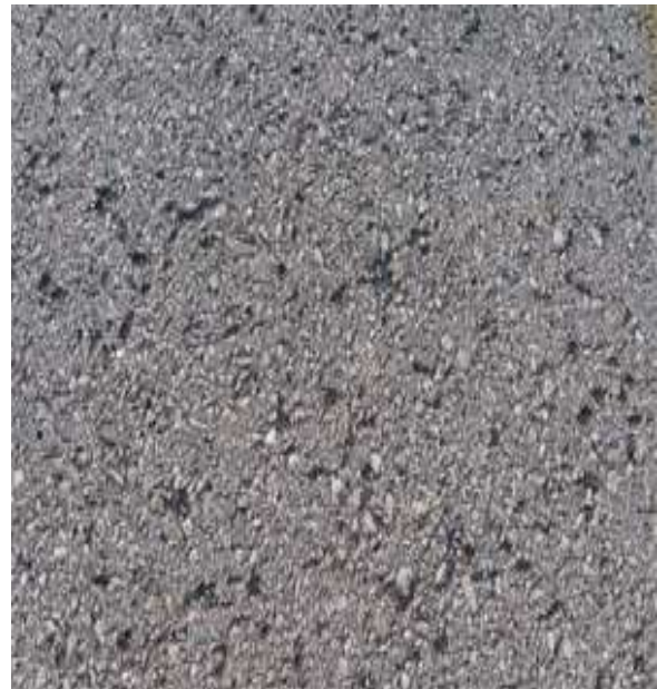
Figure 14 Medium Severity Raveling
