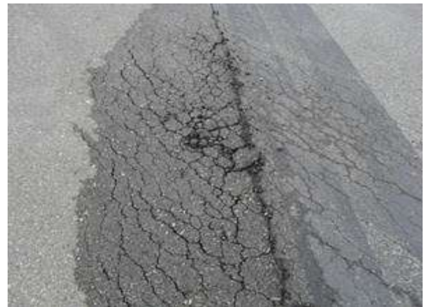
Figure 3 High Severity Alligator Cracks
