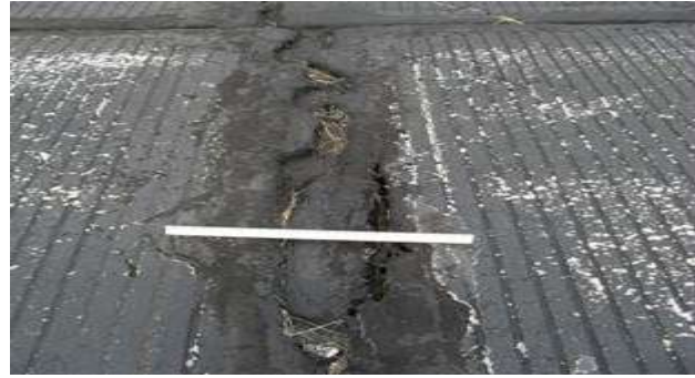
Figure 9 High Severity Joint Reflection Cracks
