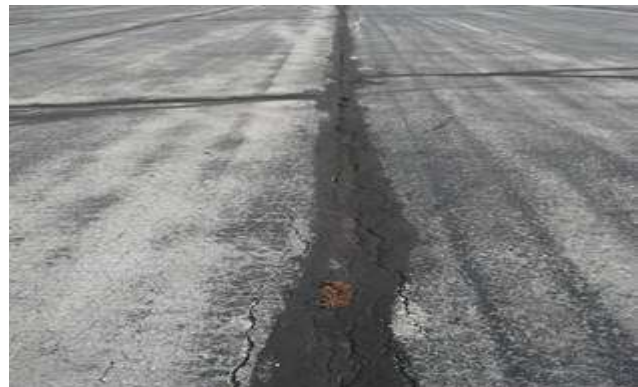
Figure 8 Medium Severity Joint Reflection Cracks
