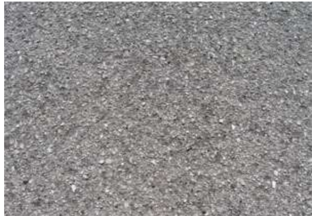
Figure 18 Medium Severity Weathering
