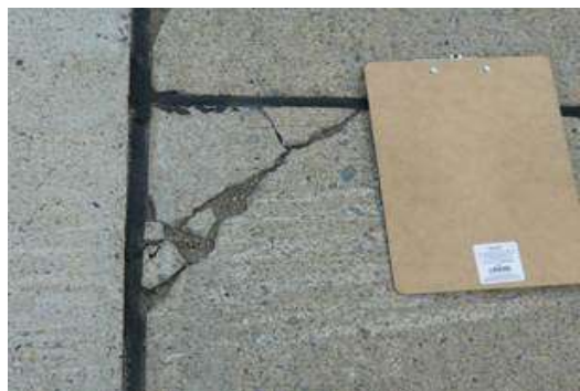
Figure 47 Medium Severity Corner Spalling
