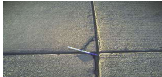
Figure 46 Low Severity Corner Spalling
