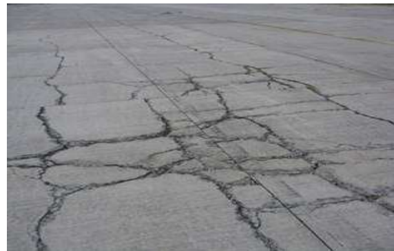
Figure 33 High Severity Shattered Slab
