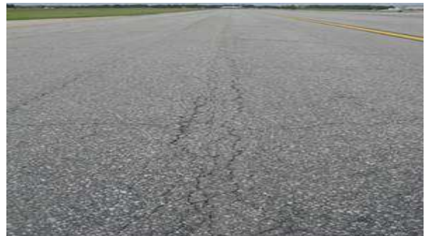
Figure 1 Low Severity Alligator Cracks
