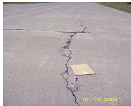
Figure 24 High Severity LTD Cracks
