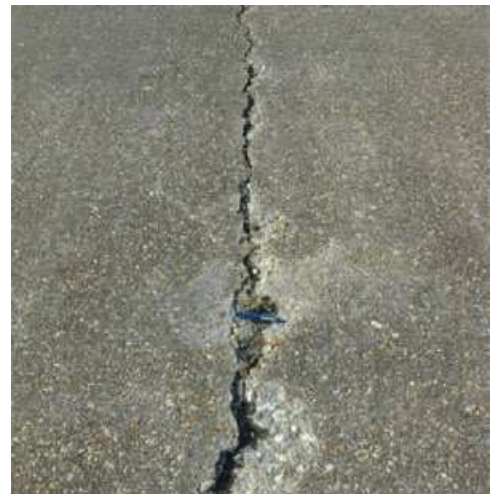
Figure 23 Medium Severity LTD Cracks
