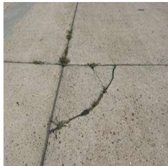
Figure 26 Medium Severity Corner Break
