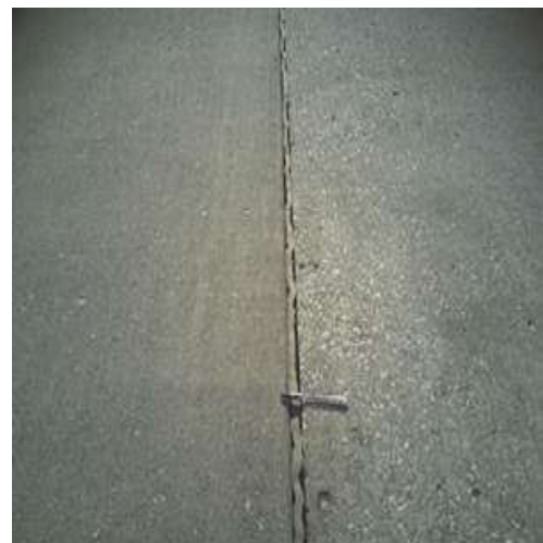
Figure 35 Medium Severity Joint Seal Damage
