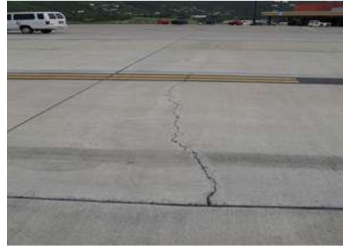
Figure 22 Low Severity LTD Cracks
