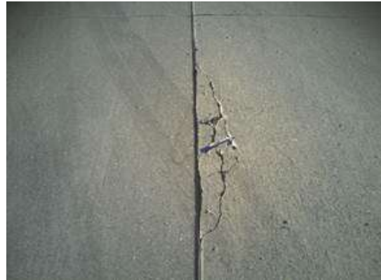
Figure 44 Medium Severity Joint Spalling
