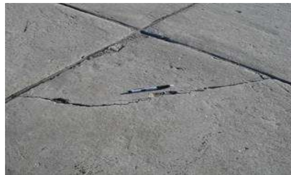
Figure 25 Low Severity Corner Break
