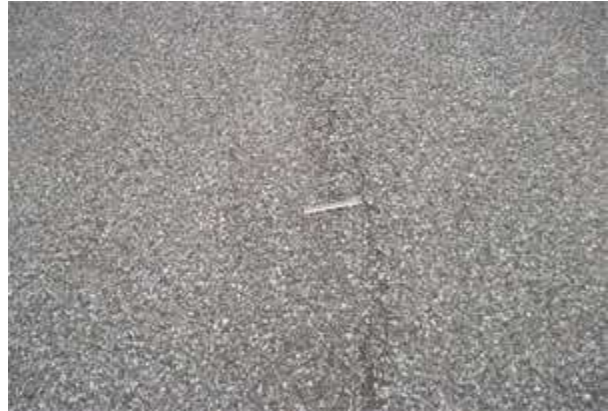
Figure 17 Medium Severity Weathering
