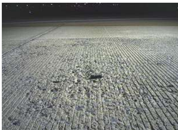
Figure 39 High Severity Scaling
