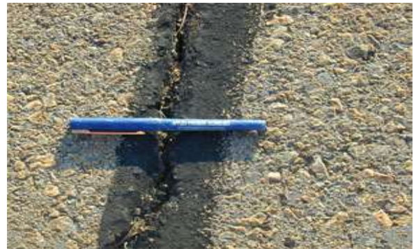
Figure 5 Medium Severity L & T Cracks
