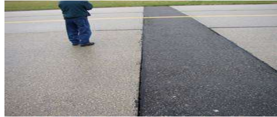
Figure 19 Low Severity Patching
