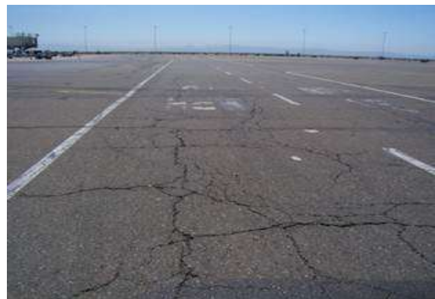
Figure 12 Medium severity of block cracks
