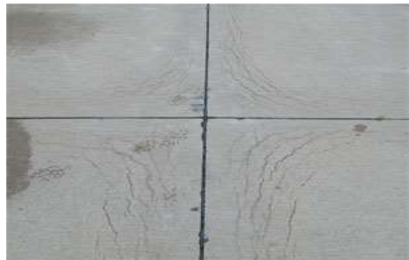
Figure 28 Low Severity Durability Cracks
