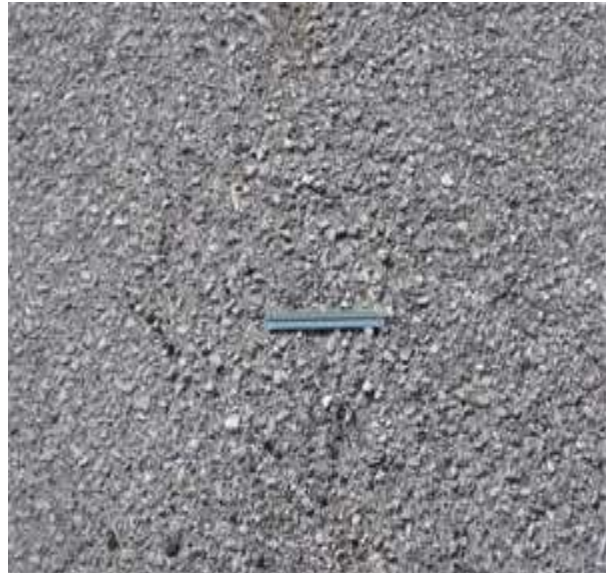
Figure 15 Medium Severity Raveling
