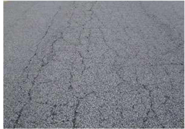
Figure 2 Medium Severity Alligator Cracks
