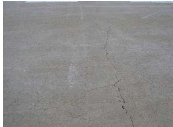
Figure 40 Low Severity ASR
