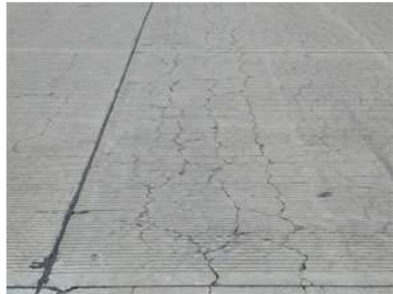
Figure 41 Medium Severity ASR
