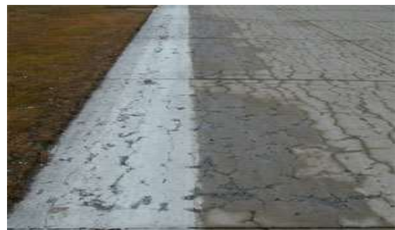
Figure 42 High Severity ASR
