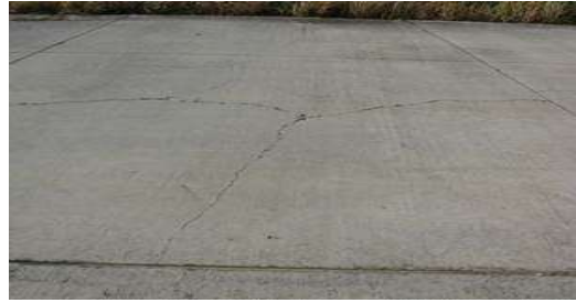
Figure 31 Low Severity Shattered Slab
