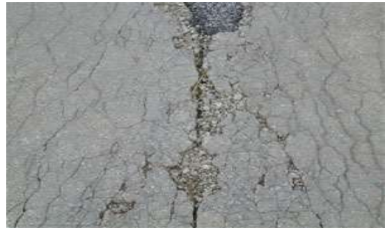
Figure 30 High Severity Durability Cracks
