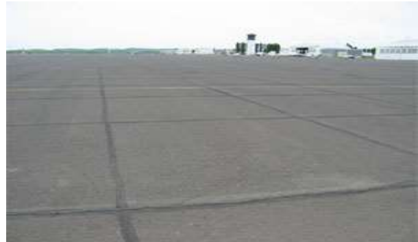
Figure 7 Low Severity Joint Reflection Cracks
