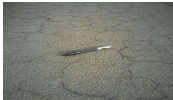
Figure 37 Low Severity Scaling
