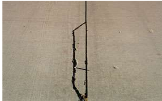
Figure 43 Low Severity Joint Spalling
