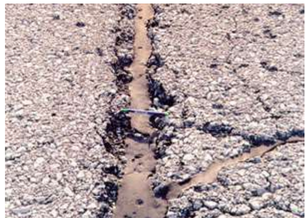
Figure 6 High severity of L & T cracks
