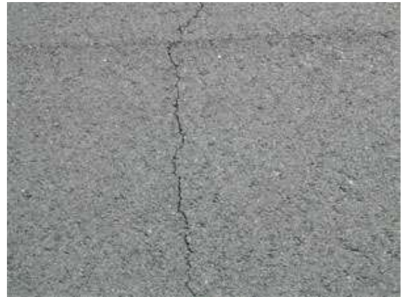
Figure 4 Low Severity L & T Cracks
