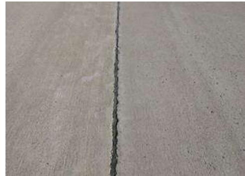
Figure 34 Low Severity Joint Seal Damage
