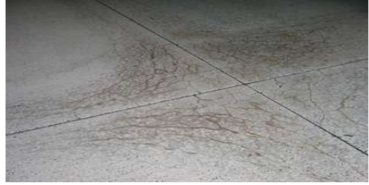
Figure 29 Medium Severity Durability Cracks
