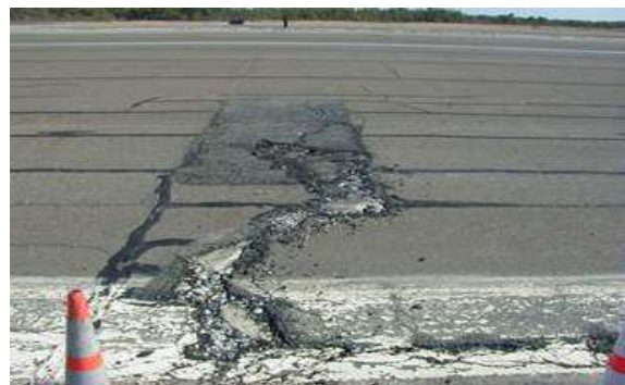
Figure 21 High Severity Patching
