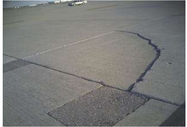
Figure 27 High Severity Corner Break
