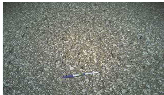
Figure 16 Low severity Weathering
