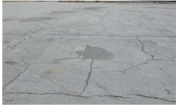
Figure 11 Medium Severity Block Cracks
