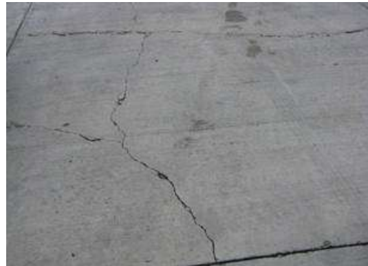
Figure 32 Medium Severity Shattered Slab
