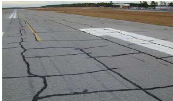
Figure 10 Low Severity Block Cracks
