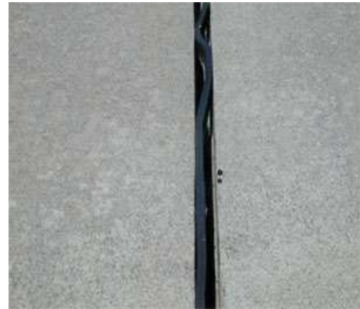
Figure 36 High Severity Joint Seal Damage
