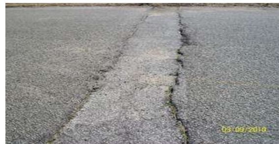
Figure 20 Medium Severity Patching
